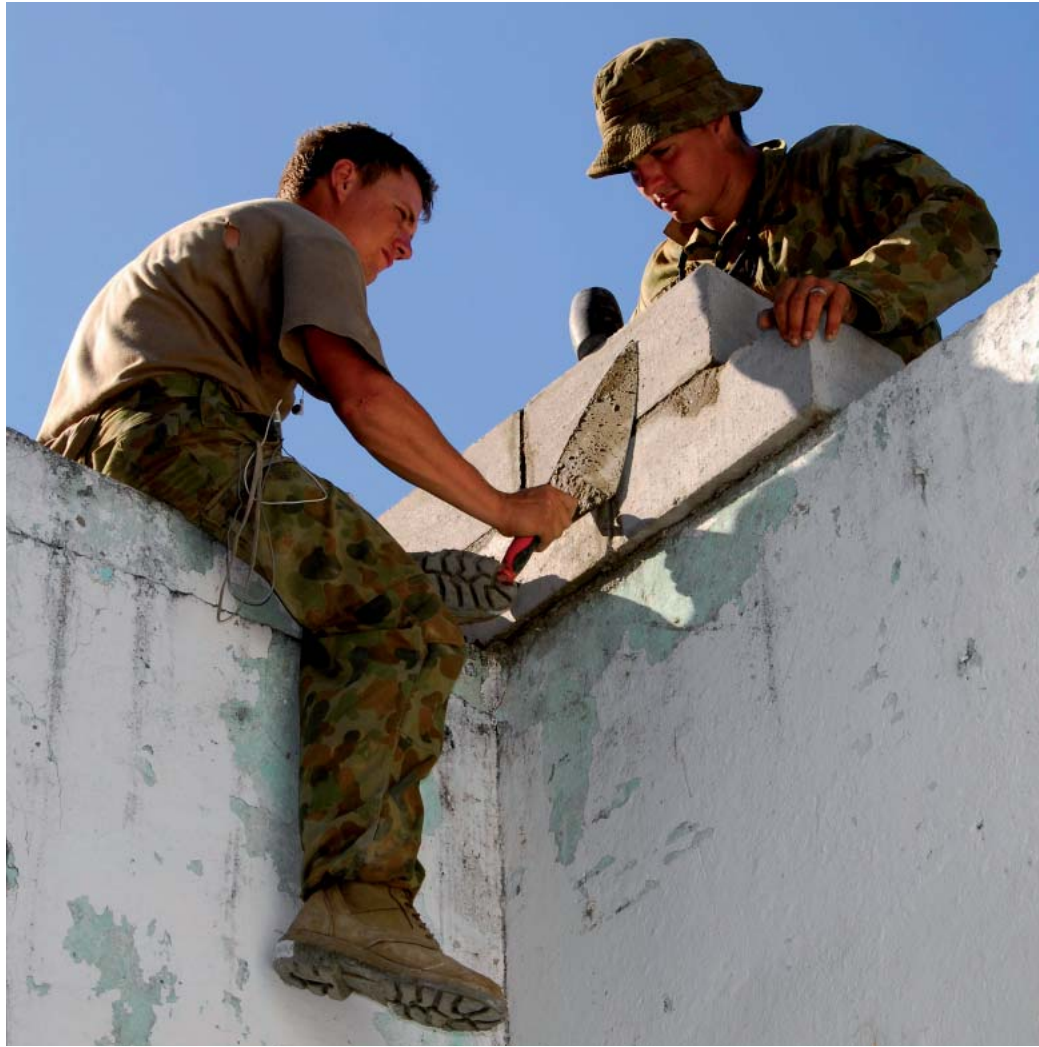
Australian Engineer Regiment sappers carry out repairs at Camp Phoenix, Dili, July 2006 Photo: Courtesy Department of Defence © Commonwealth of Australia 2009
